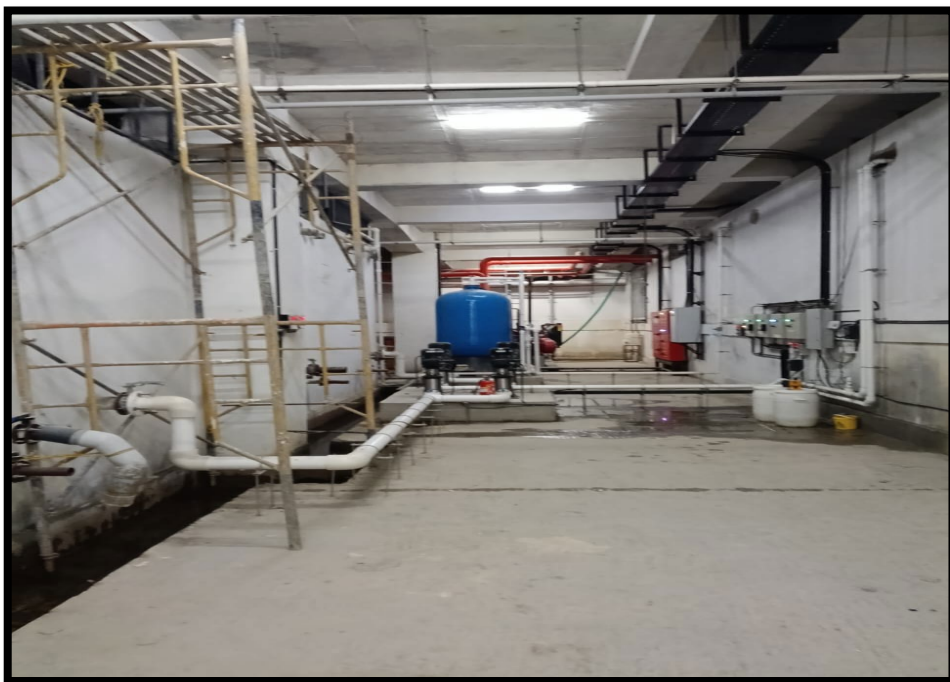
Rain water tank
